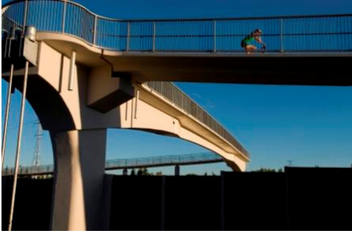
Figure 7. The bridge. The drop in girder is the part with the thin web and wider flanges than the abutments which stretch out from the column's construction.
